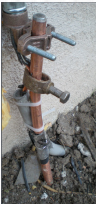
Grounding Electrode Connection
